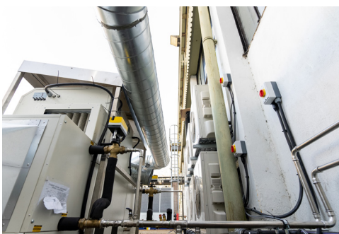
External plant area and ducting for HVAC system
