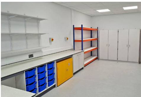
D & T prep room with hazardous substance storage
