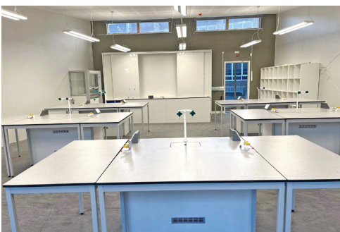
Science lab with serviced bollards & loose tables
