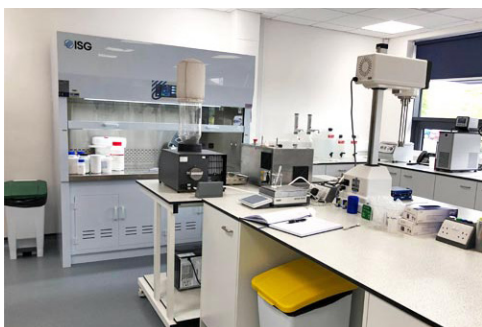
Recirculating fume cupboard with steel liner
