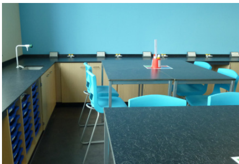
Trespa benching with perimeter services
